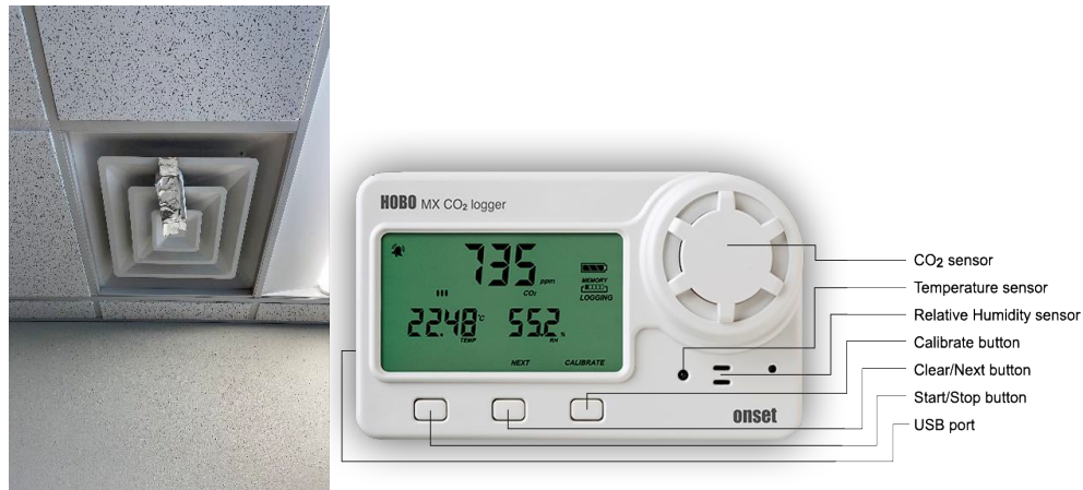
Figure 2-17. HOBO CO 2 Sensor Installation
