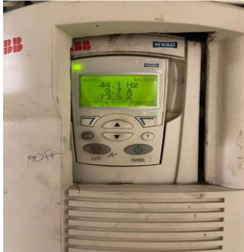
Figure 2-12. Variable Frequency Drive (VFD)
