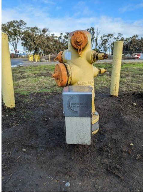
Figure ES-3. Wet Barrel Hydrant, as Retrofitted with hydrant.AI Sensor Station at NBVC Port Hueneme Demonstration Site.
